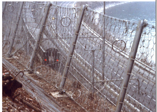
Figure 1. A Wire-net rockfall protection system.
