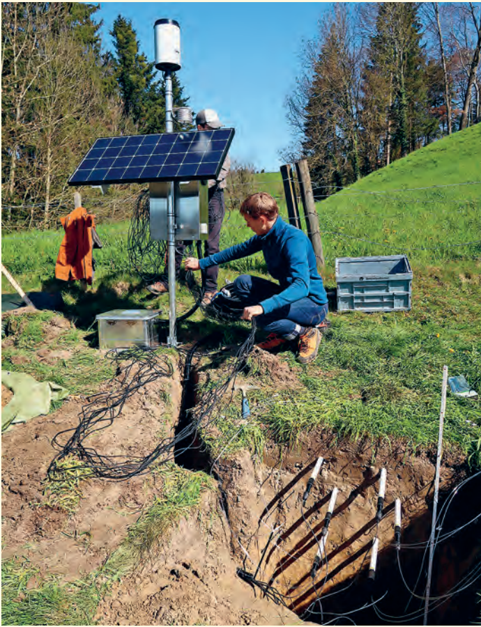
Installing a soil wetness monitoring station near Ranflüh (Canton Bern). Here a researcher is wiring the sensors placed in the soil profile to the data logger.
